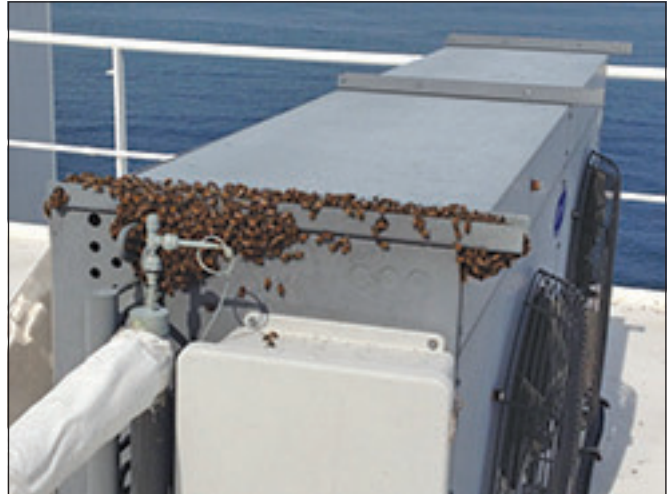
Figure 5. Bee swarm on air conditioning unit aboard USNS Comfort (TAH-20) in port in Acajutla, El Salvador. Photo courtesy of LCDR J. Dunford.
